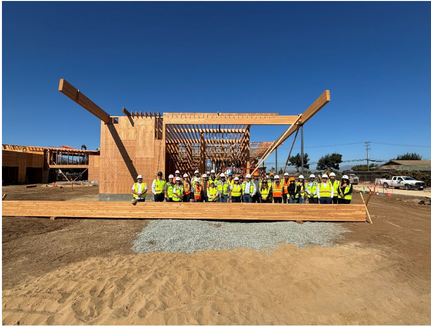
Topping out ceremony, Celebrating installation of the last structural beam at Building A.
